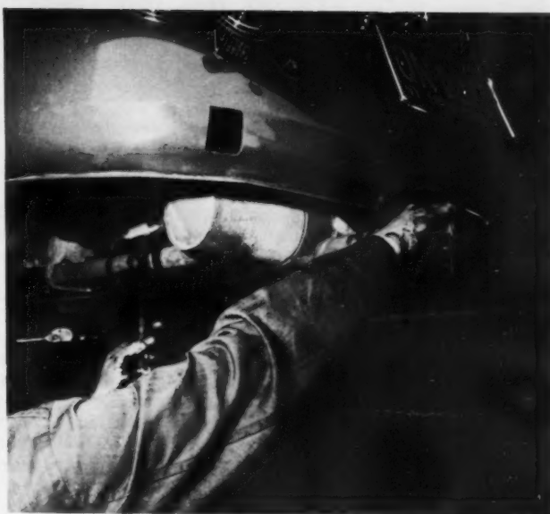
Using a rubber mallet, tap the old muffler gently at either end until it drops free from both pipes and upper flange studs. Be careful not to damage or burr the studs in any way.
